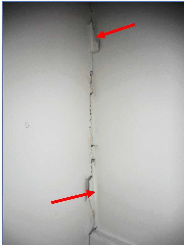
BEDROOM CLOSET WALL TO WALL INTERSECTION SEPARATION
