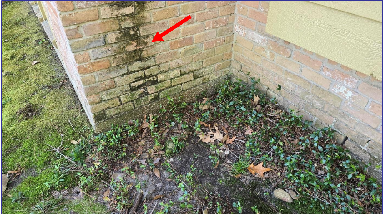
DARK STAINS ON BRICKS DUE TO CHRONIC WATER CONTACT
