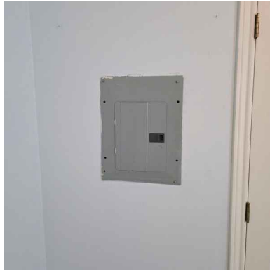
Sub-Panel Manufacturer: Eaton
