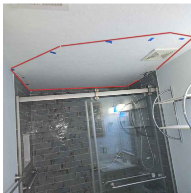
Primary Bathroom - most affected area
